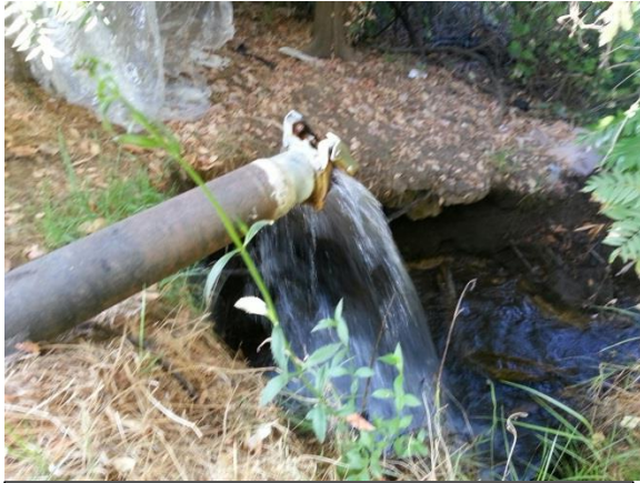
Figure 3. Outlet pipe into Bushy Lake from Cal Expo. Photo by Julian Fulton.
